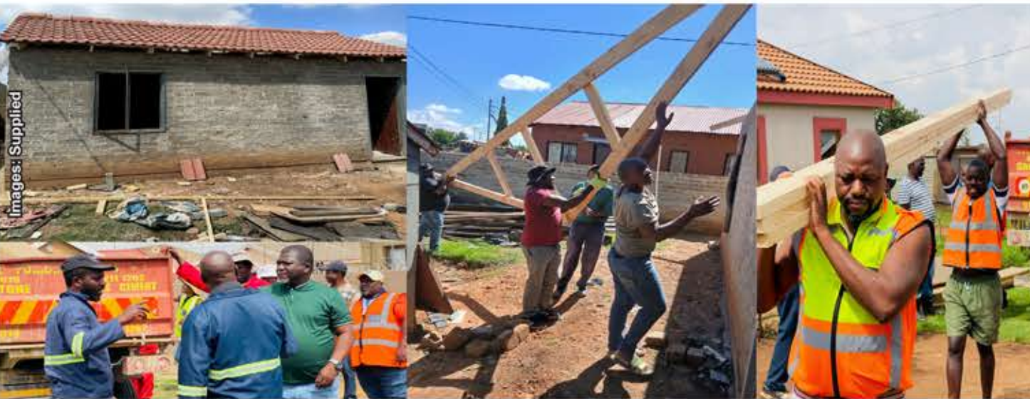
RESTORING DIGNITY THROUGH UNITY: Drieziek residents, joined by local leaders, come together to install a roof for Sefuli's unfinished RDP house, ending years of hardship and exposure to harsh conditions
